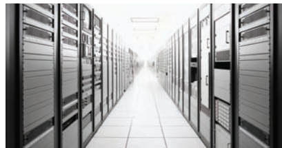
IP-based access control makes sense in IT server rooms, where mini readers can keep each IT cabinet locked.
